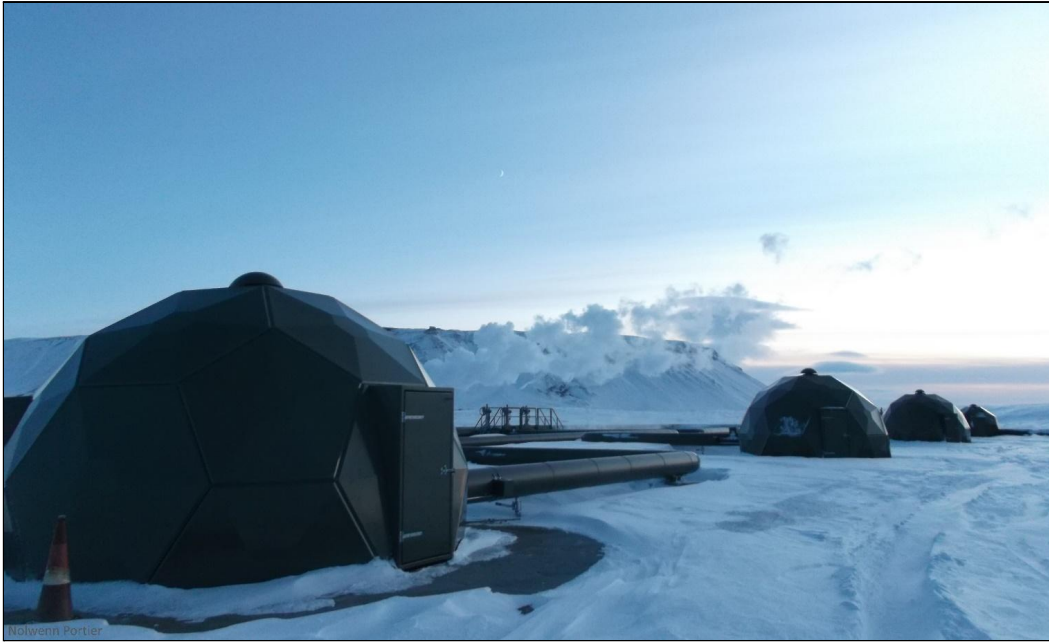
Injection well at the Theistareykir geothermal power plant (Iceland)
